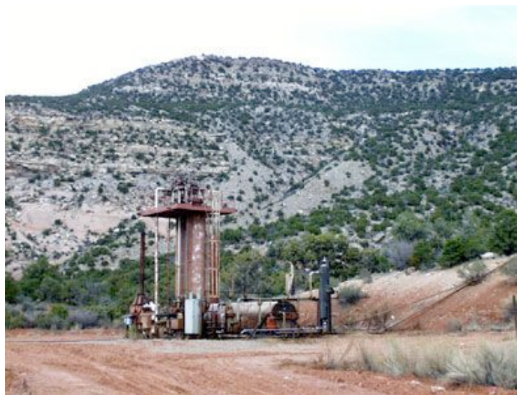
CO 2 well in Canyons of the Ancients National Monument. Photo courtesy of the BLM.
