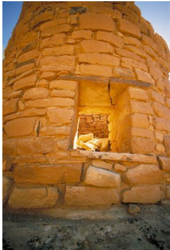
Stabilized tower in Canyons of the Ancients National Monument. Photo courtesy of the BLM
