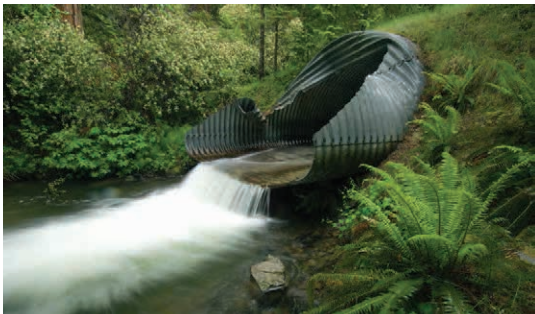
Culverts like this create fish passage barriers for native fish and can create major sediment problems when they blow out during flooding
